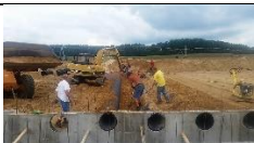
Air tubes are being installed in Kitchen Farm construction project. Photo credit: Dracht Construction
